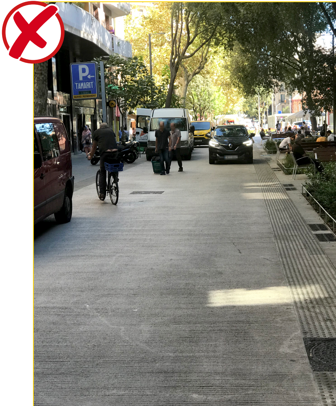
Image 29. Incorrect placement of warning strips.
